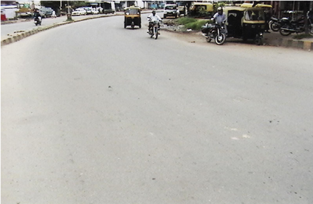
The same stretch of road unaffected by prolong pooling of water
